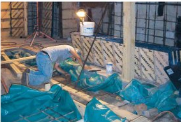
Figure 3. Before the walls could be poured, the waterproofing subcontractor installed MiraDrain and MiraClay membranes all the way to the top of the excavation (top left), then covered the exposed dirt at the top with a poly vapor barrier (top right). He also spread poly over the dirt floor in preparation for placing the slab (above).
